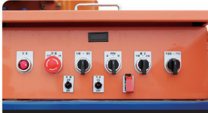
MAIN CONTROL PANEL BOX
